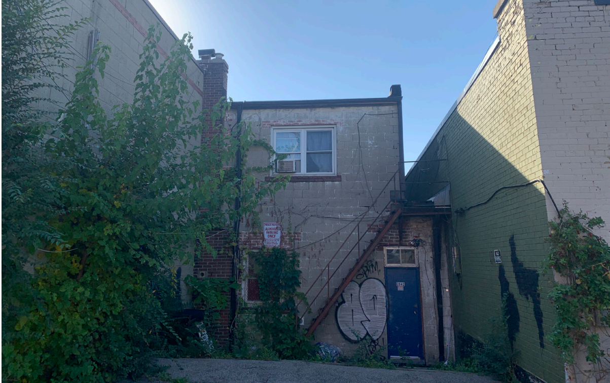
Figure 9. Partial north elevation of the Site looking south from the rear laneway (ERA, 2022).
